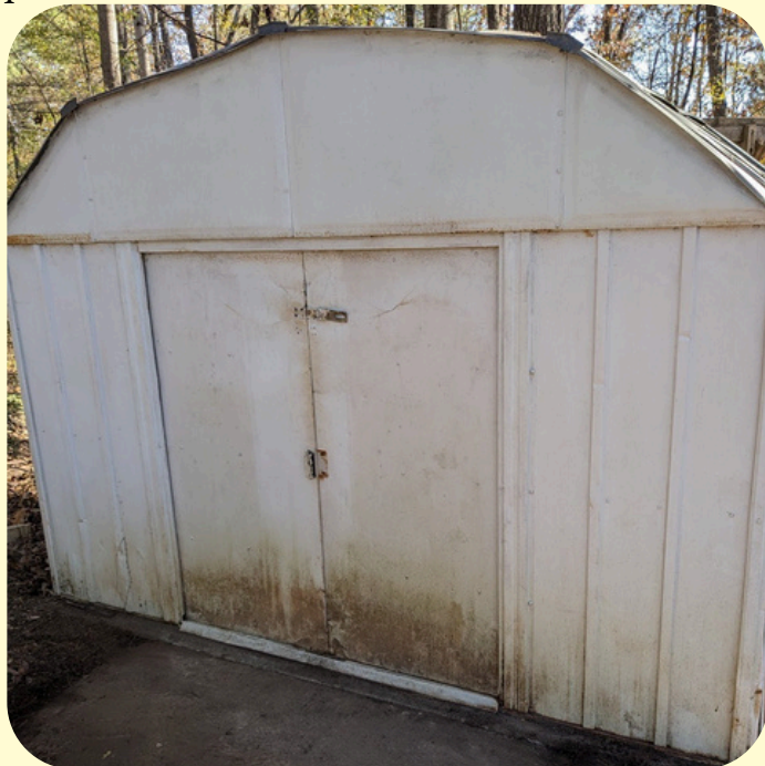
I found a concrete pad in front of the shed! Still needs cleaning, perhaps some paint.
